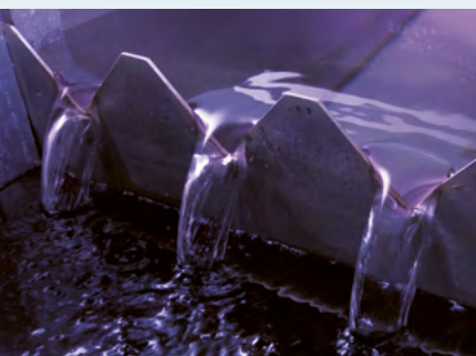
Disinfection of water using UV light.
